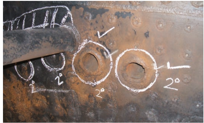
Overfire jets are shown here in the firebox of RFIRT 107. The demodernization over time by shop crews is shown as the left two jets have been seal welded with stay bolts placed in the centers. - S.T. McMahon
